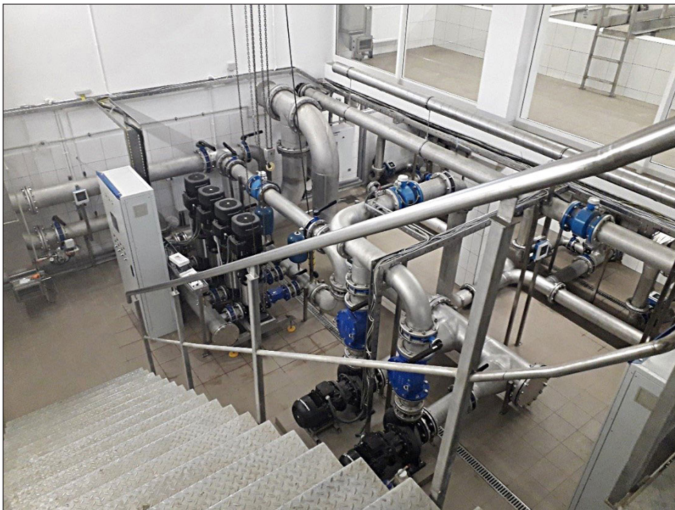
Figure 2. Sample photo from WTP after modernization – pump hall
