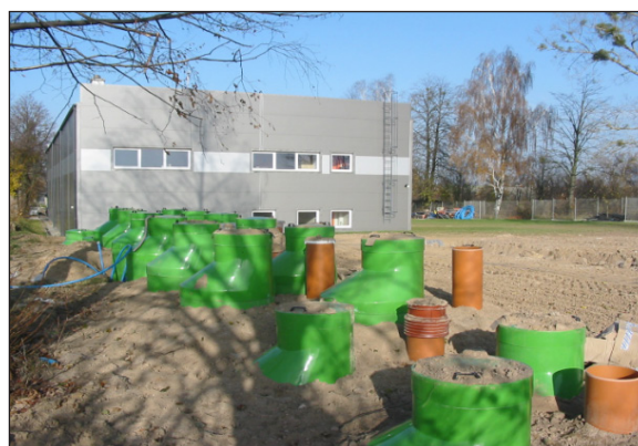
Figure 12. Research installation built in pilot plant scale
