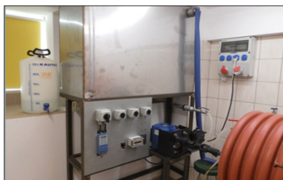
Figure 11. Fundamentals of Technology Department Laboratory – control panel of the rotating biological contactor with bi-directional longitudinal flow
