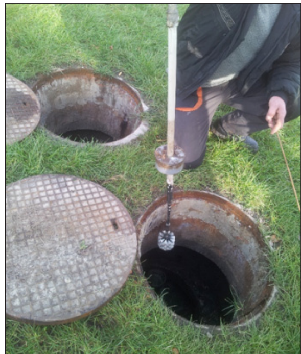
Figure 8. Manhole cover with float system being controlled
