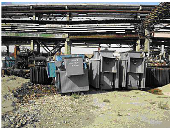
Figure 1. The oiled power transformer
