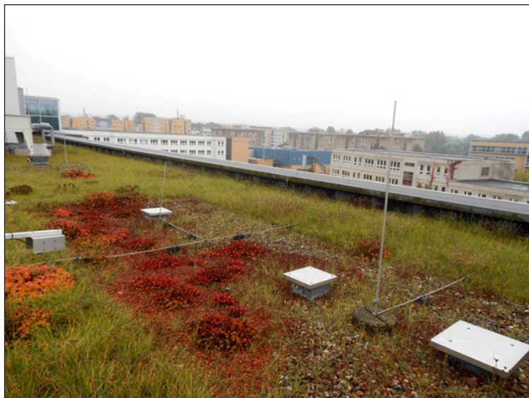
Fig. 4. Neubrandenburg, Germany – the roof of the Hochschule building with a rainwater system
