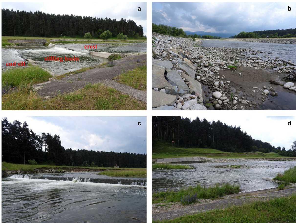
Photo 1. Channel section with grade control structures on the Biały Dunajec in the city of Nowy Targ: a – GCS, b – recreated and newly reinforced riverbank, c – damaged bank reinforcement and partly eroded GCS's crest, d – GCS covered with debris
