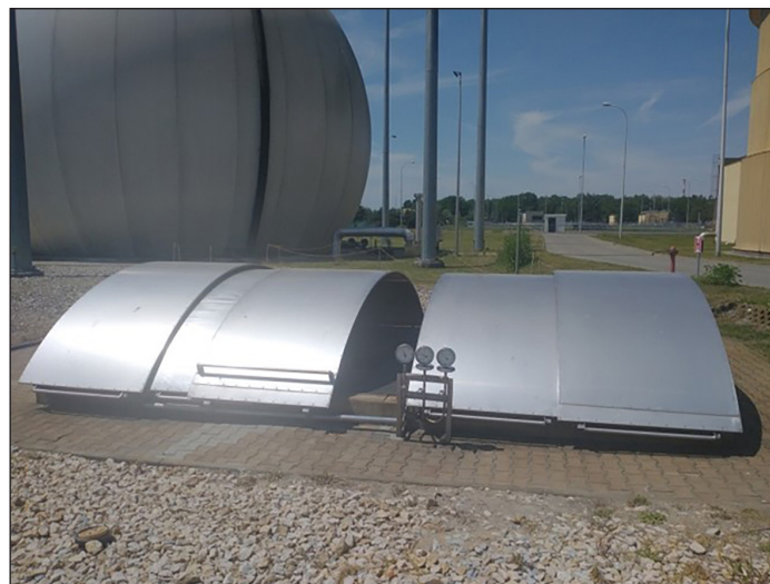
Figure 1. Biogas desulphurisation plant at the wastewater treatment plant in Tychy
