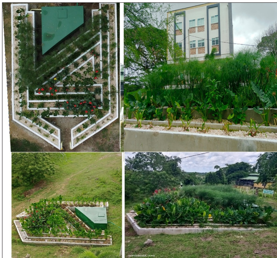
Figure 2. Full-scale ornamental constructed wetland
