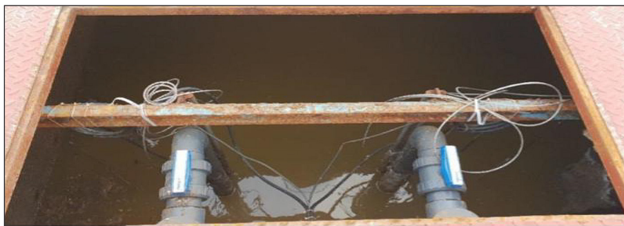
Figure 4. Wastewater collection and distribution room in wastewater treatment plants
